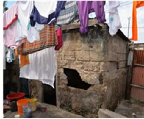
Water eroded walls, Pakacha
